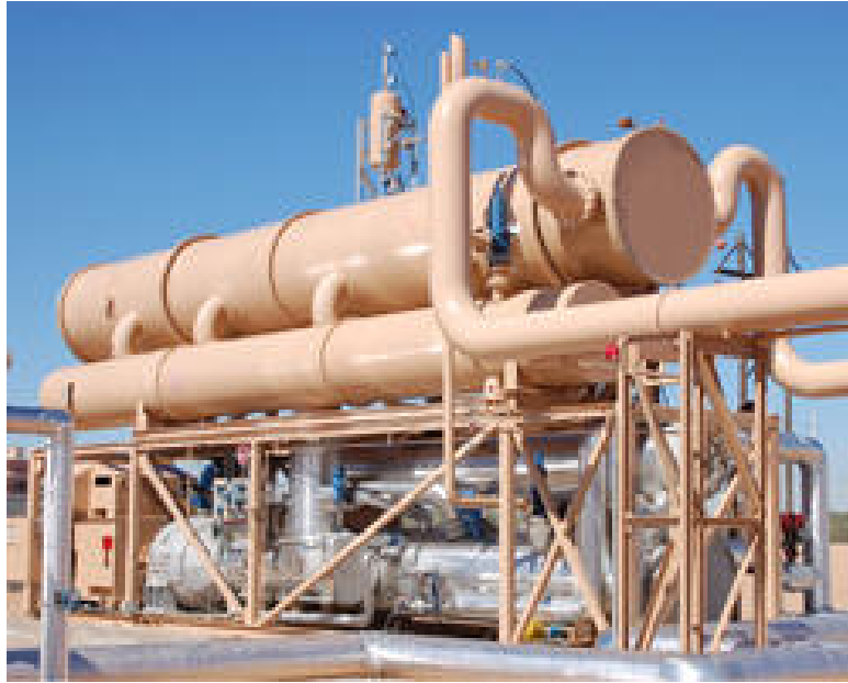
Figure 2.13 Organic Rankine cycle power plant in Saguaro, Arizona [75]
