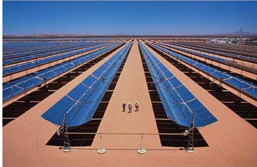
Figure 2.3 Parabolic trough solar collectors [10]
